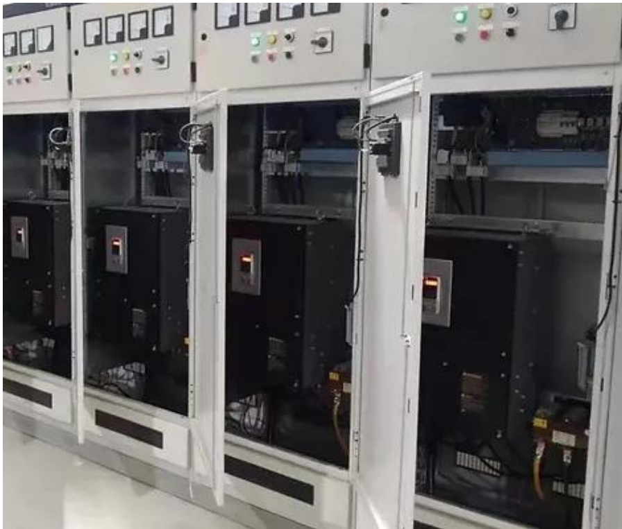
120HP AS180 series VFD installation for a water supply and treatment plant, replacing the original soft-starter system. PID control was programmed for automatic speed regulation, excellent control performance and to make the pump system operate efficiently with minimal manual intervention.
