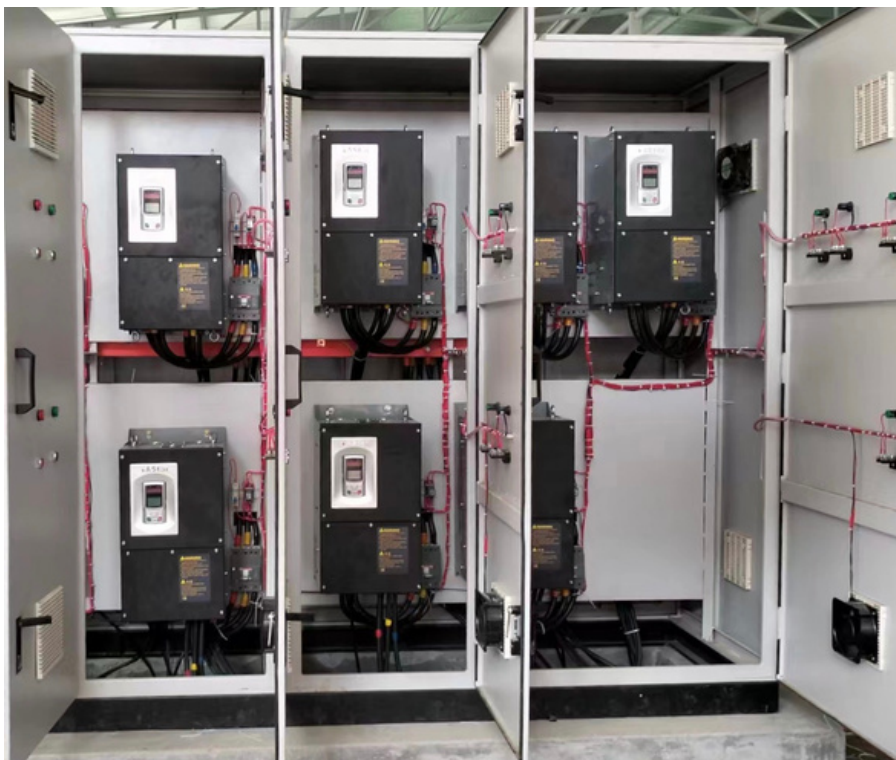
AS450 Drive installation for a water pump control system to provide maximum flow at optimal efficiency. The drives provide extensive diagnostics with regards to maintenance of water pressure and simplifies the complexity of the entire flow control system via the built-in PID controllers.
